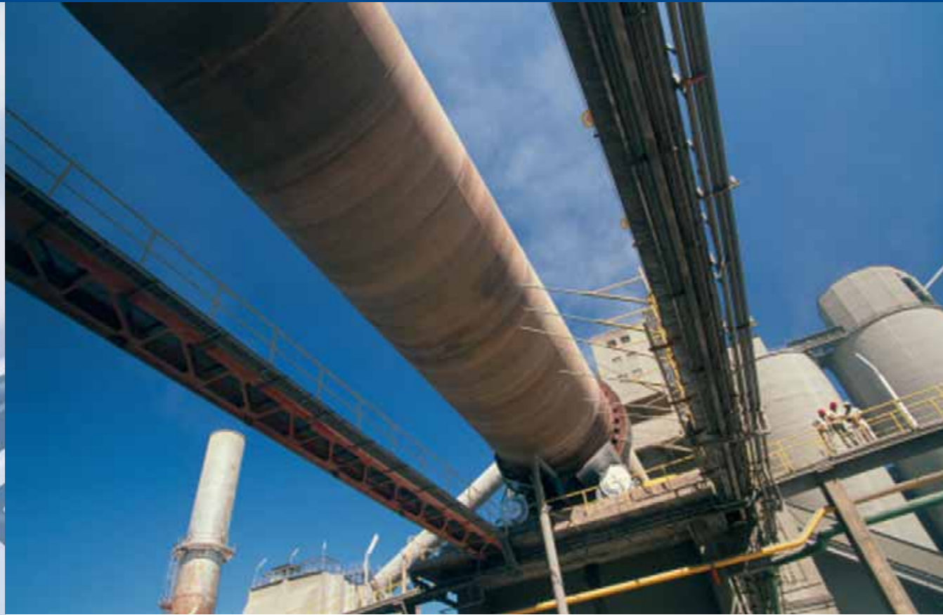
Rotary Kiln with DC-Motors
